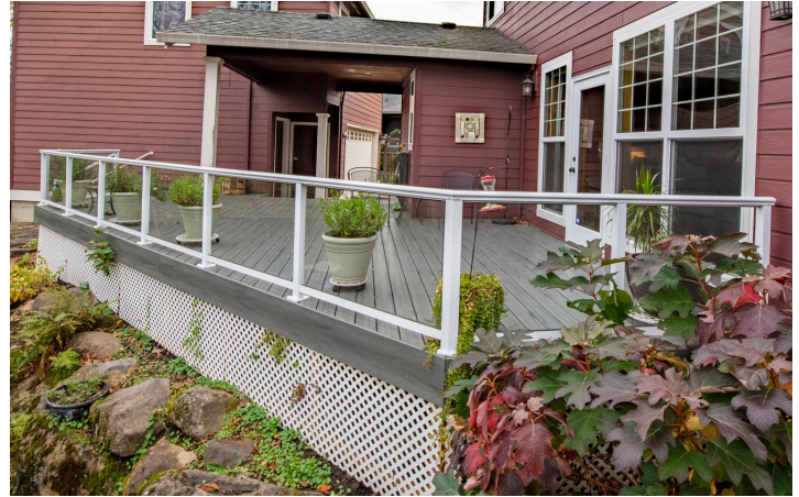
Set against a wooded backdrop this deck was completed with Elliptical Top TR999 Railing System and paired with glass infill for optimal wind protection.
